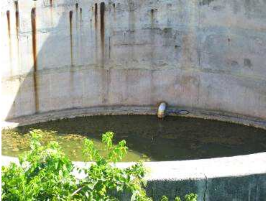
Sea Water Storage Tank Internals
