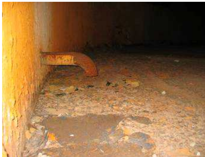
Corrosion of Decommissioned Water Storage Tank Floor
