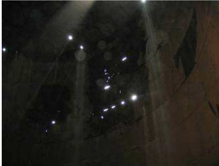
Corrosion in Decommissioned Water Storage Tank Walls
