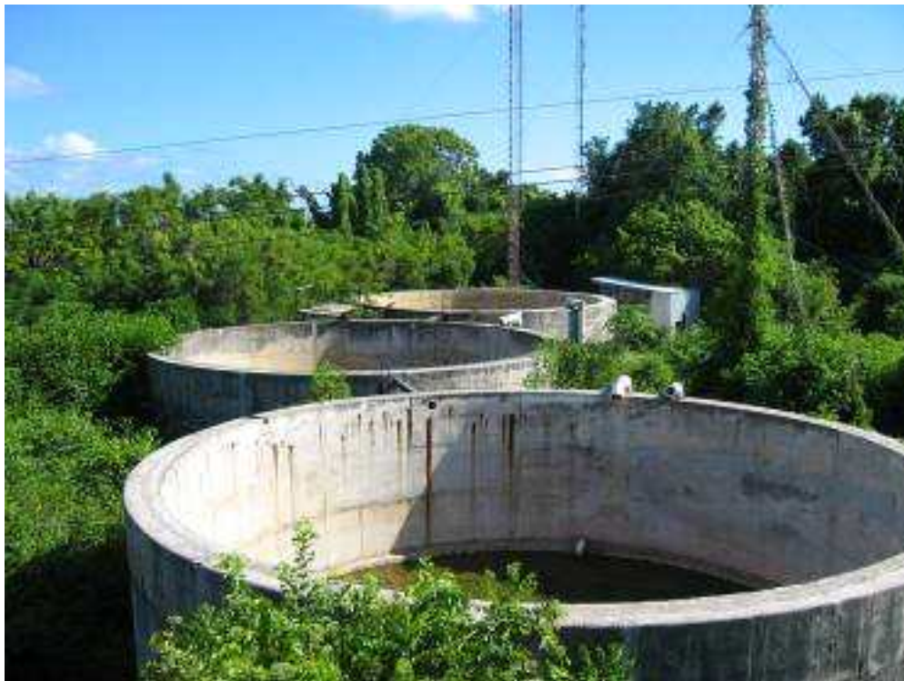
Sea Water Storage Tanks at Command Ridge
