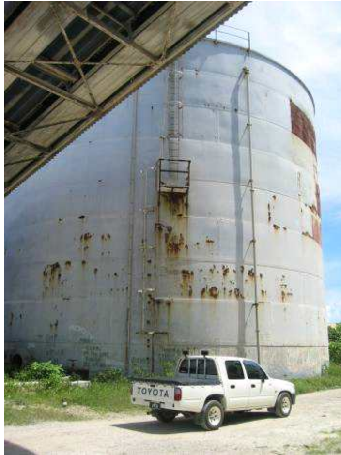
Potable Water Storage Tank B13
