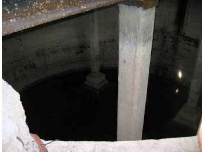
Rain Water Collection Tank
