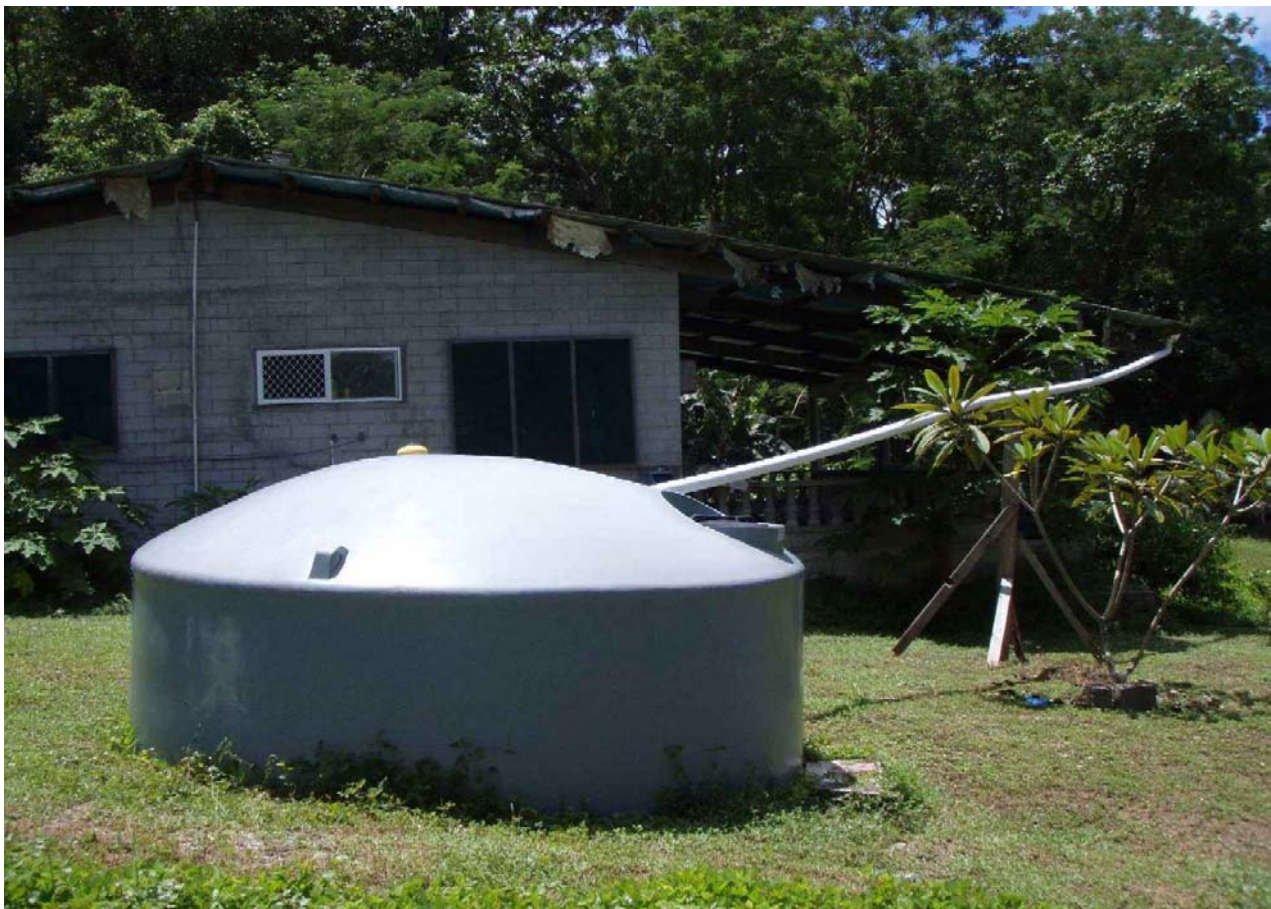
Plastic water storage tank emplaced partially below ground level, Buada, Nauru.
