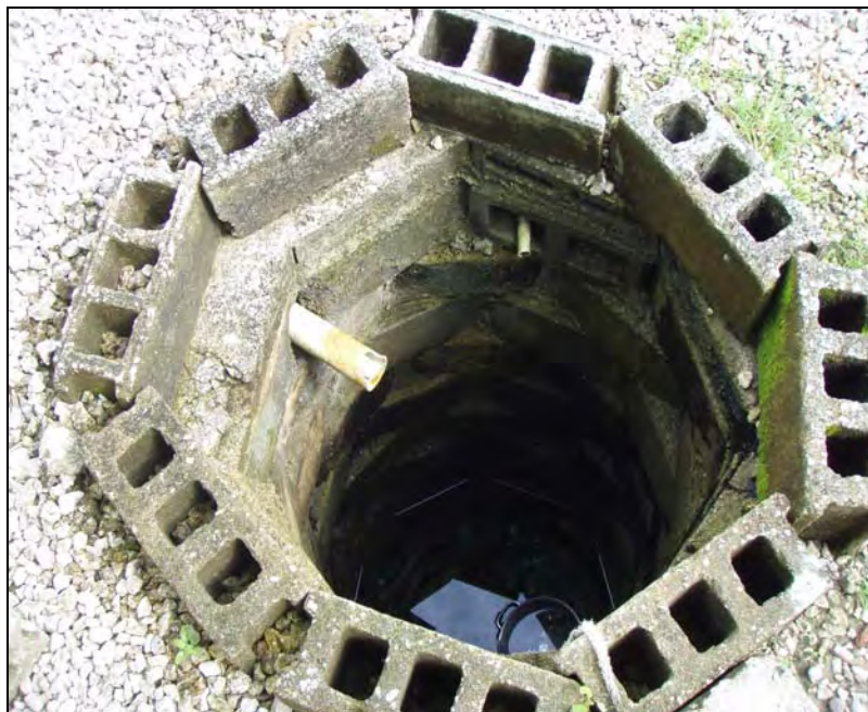
Figure 27. Alternative supply well, Buada District..
