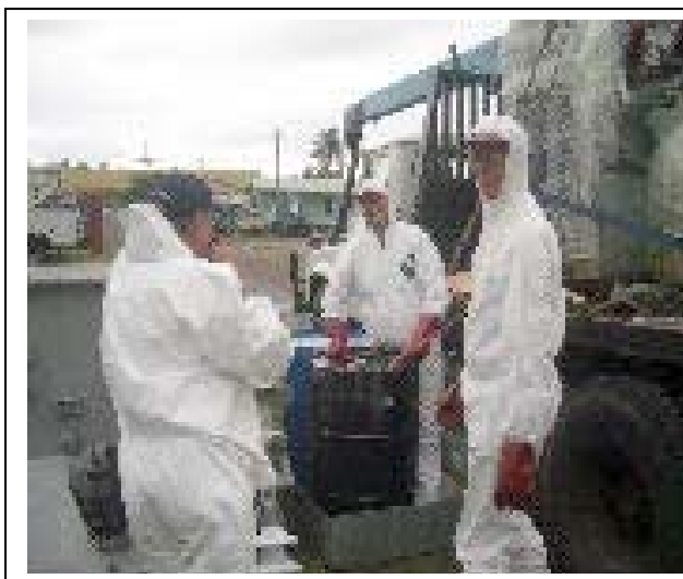
Figure 3: Two AMC consultants and Project Coordinator POPs draining PCB-contaminated transformer oil from Savaii. Photo: MNRE.
