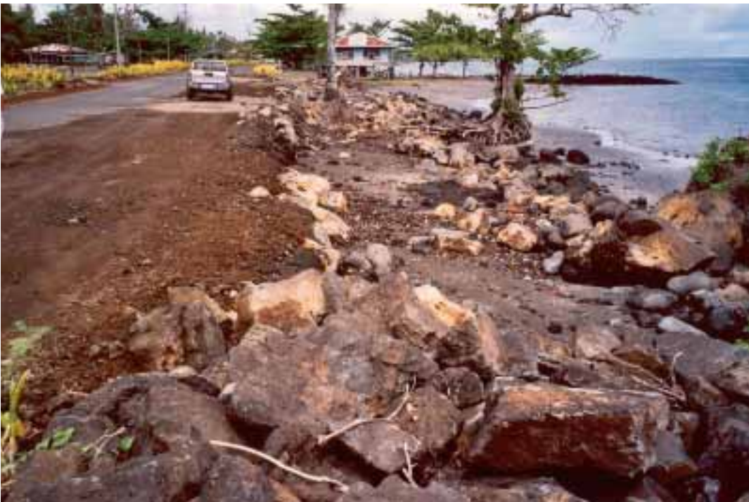
Figure 7. Road damaged by Cyclone Heta, Savaii, Samoa
