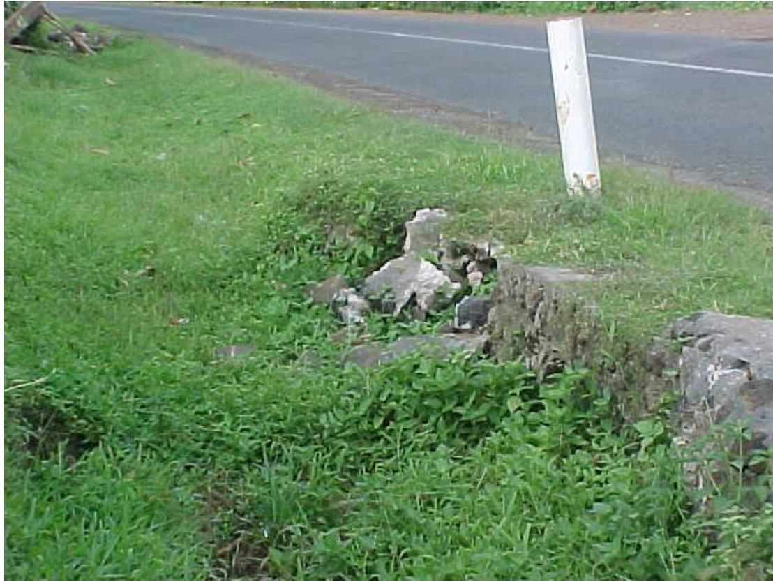
Blocked drain behind road at Saletagaloa.
