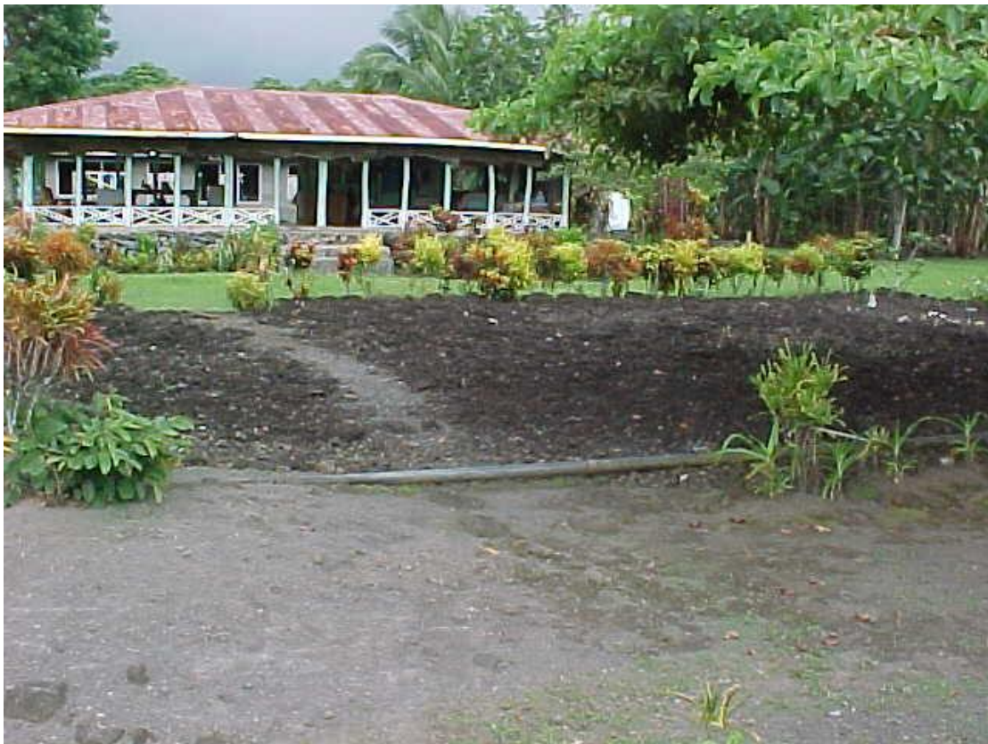
Flood area behind road at Vai'afai caused by culvert outlet invert being lower than surrounding ground levels. Exposed galvanised water pipe to be replaced by new PVC pipe under the EU Rural Water Supply Project.
