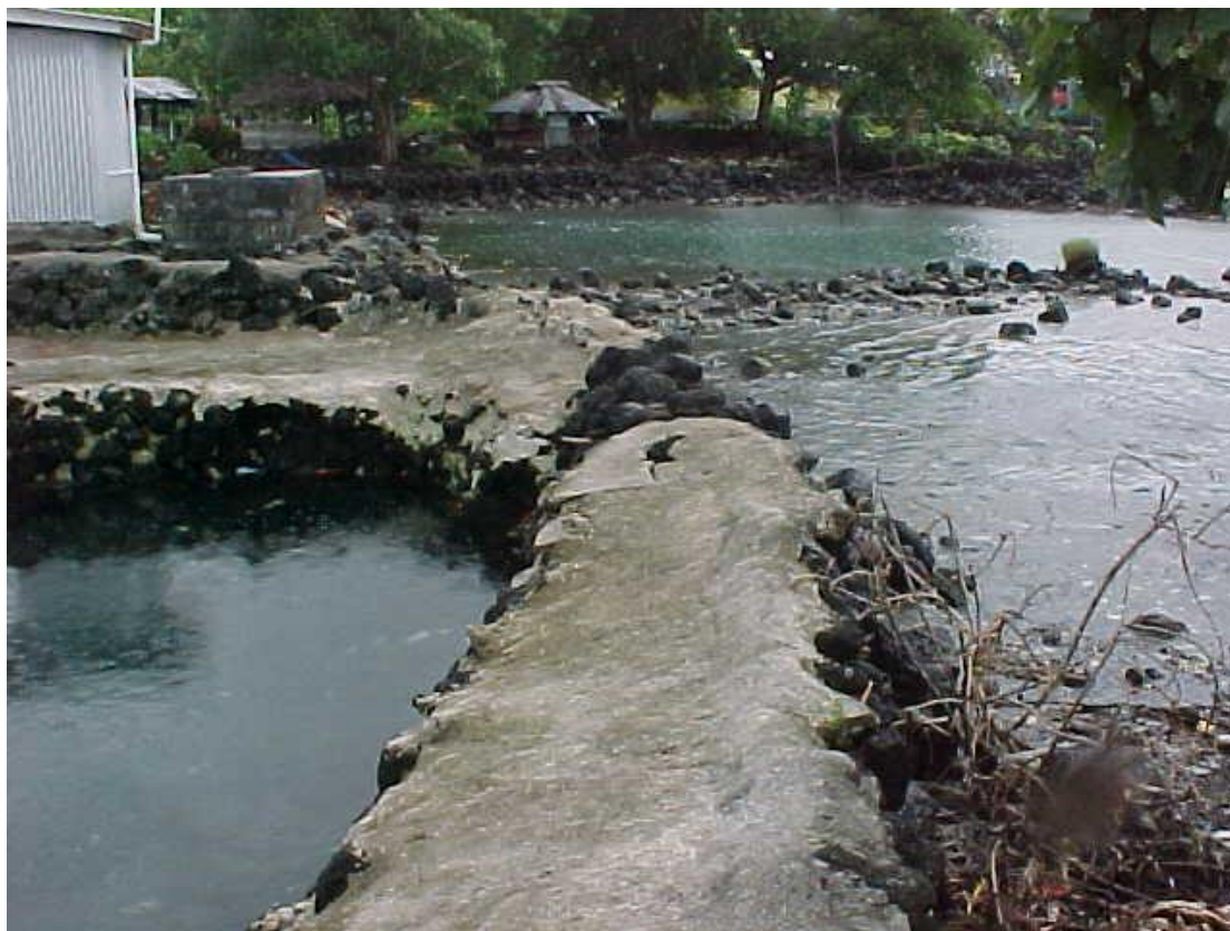
Vaitele Pool wall. Small rock construction and location results in high risk and susceptibility to damage.
