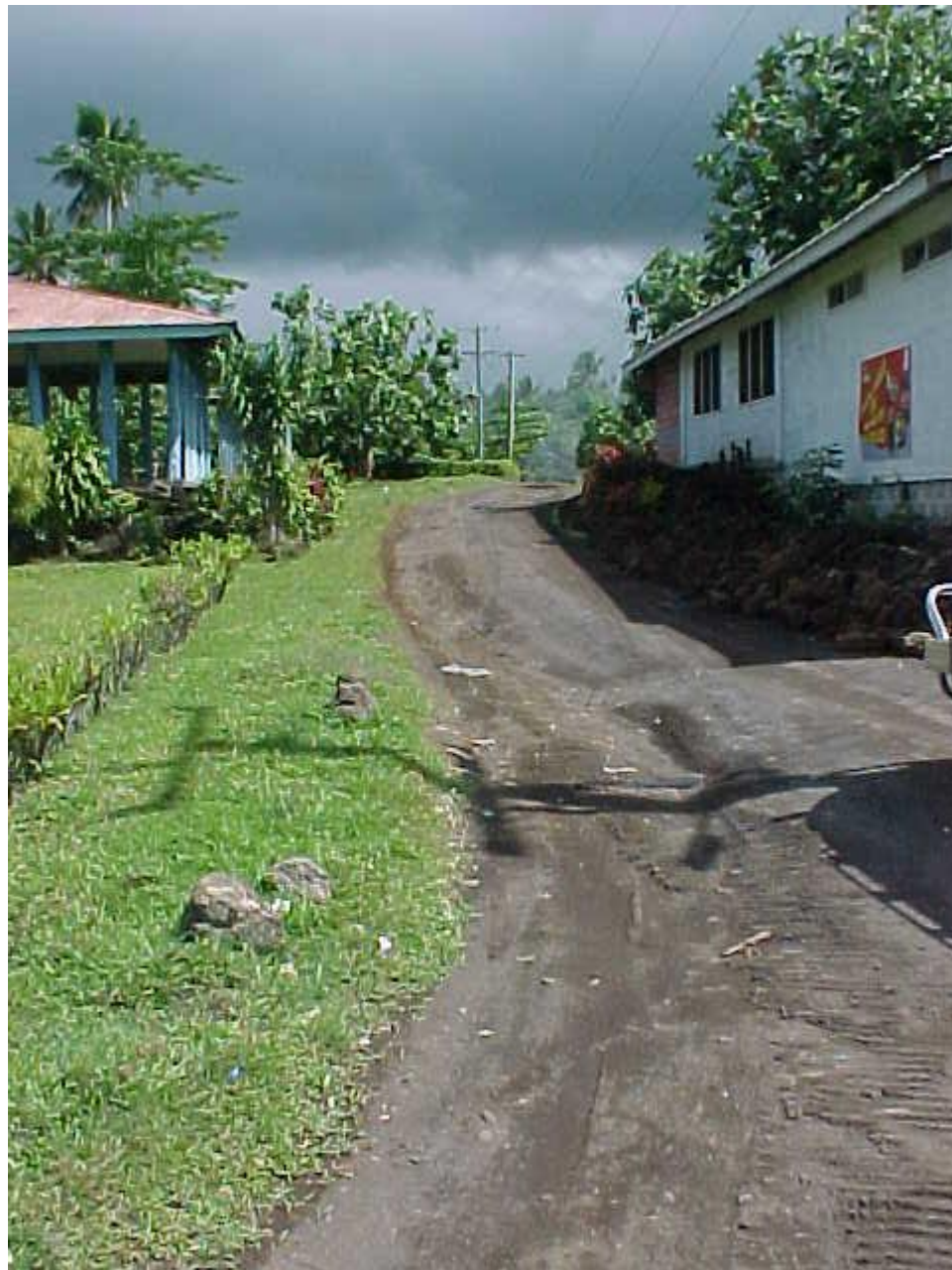
Work road intersection with Main Road showing scour along left hand side.
