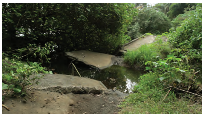
Collapsed bridge on Epi's west coast Photo: PACC
