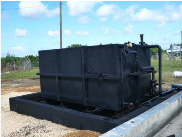
Photo 14: Used oil storage tank connected to the generator waste pit
