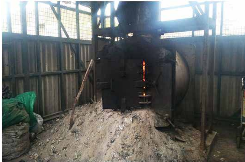
Figure 12: Incinerator at the Jackson's International Airport, PoM
