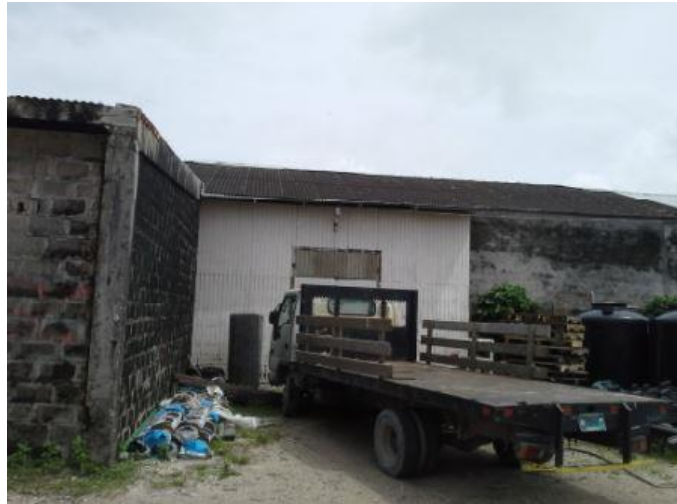
Photo 3: Asbestos roof cladding at Ace Hardware
