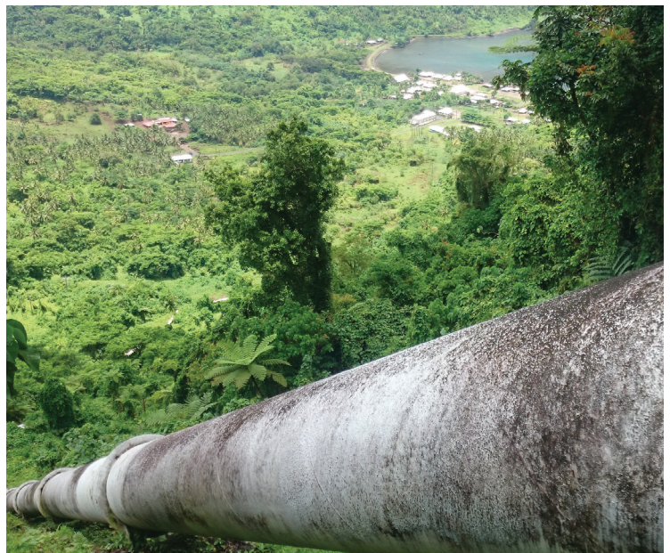
The pipe (penstock) that carries fast-flowing water from the dam to the hydropower station to generate energy.
