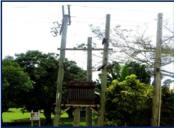
Photo 9: Old pole mounted distribution transformer on TPL distribution grid in Vava'u
