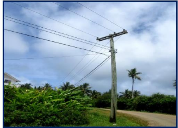
Photo 10: Existing overloaded wooden pole on the verge of felling in Vava'u Island
