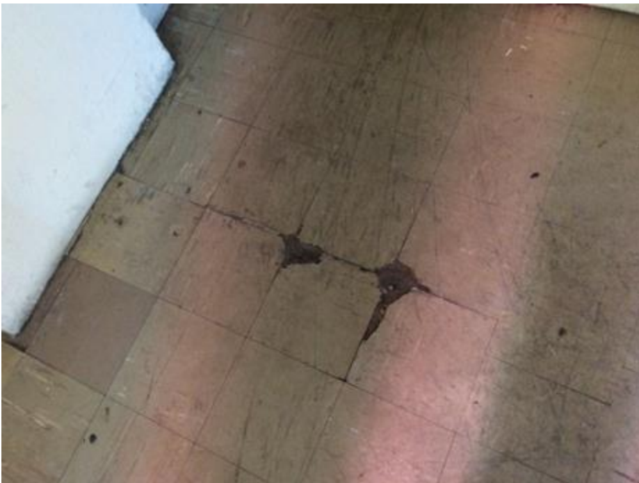
Photograph 2: Damaged ground floor vinyl floor tiles sampled 16 July 2014.
