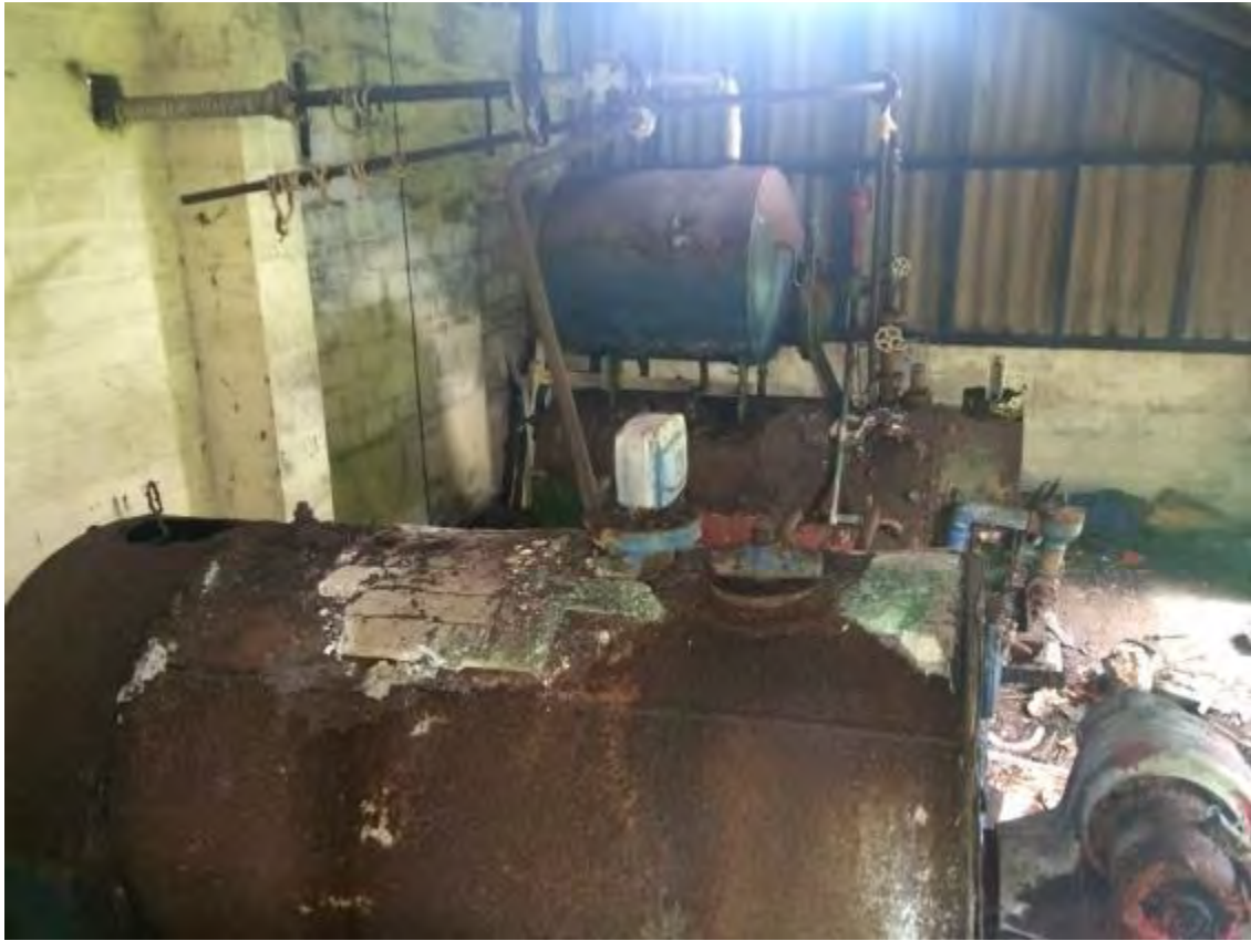
Photo 13: Residential property 18, boilers with ACM lagging
