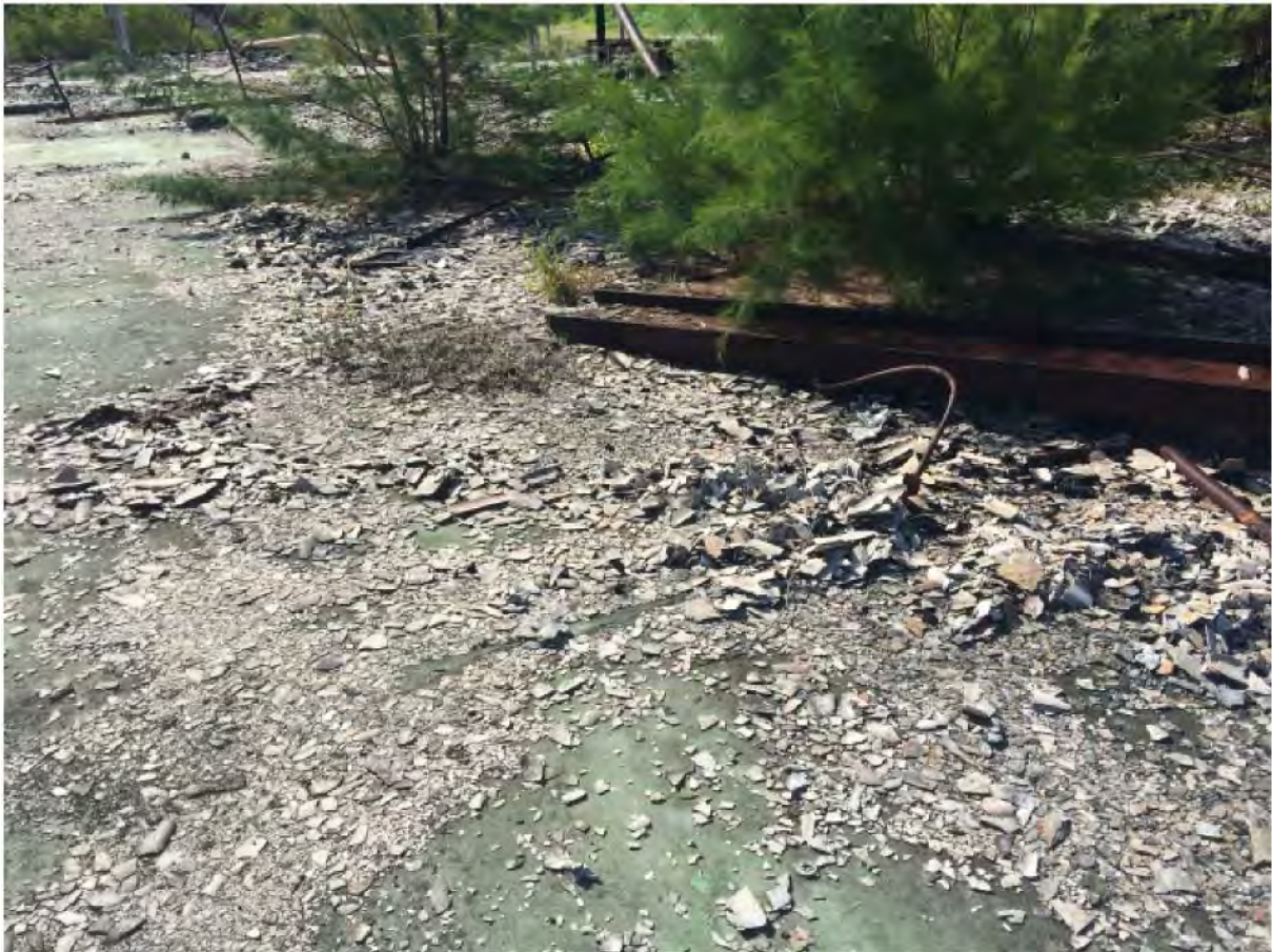
Photograph 4: Warehouse 4; view of pacm debris.
