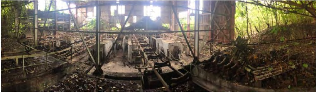
Photograph 9: Former phosphate processing plant. In disrepair with significant pacm scattered across entire site.
