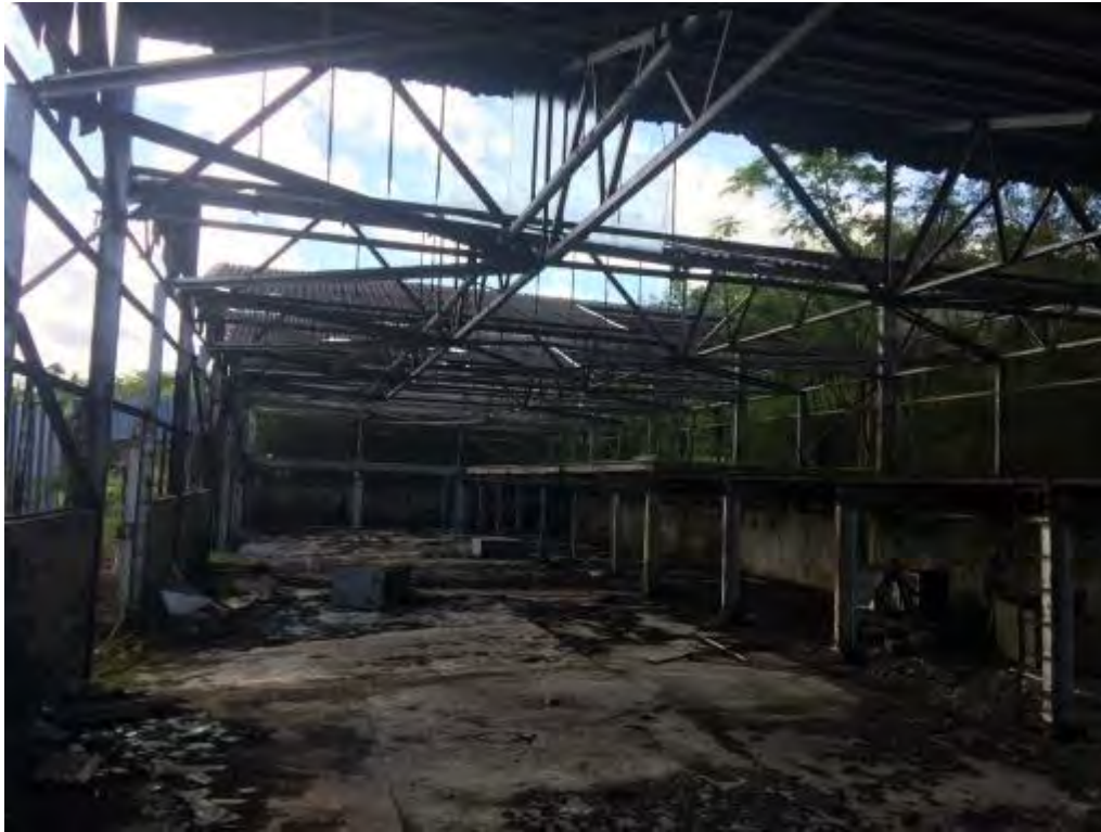
Photo 22: Warehouse 3 – badly damaged ACM roof and walls.
