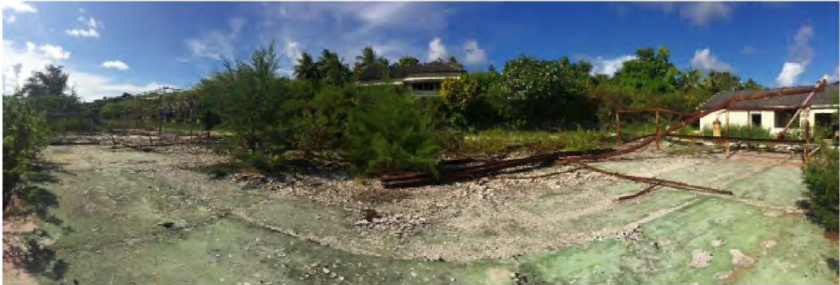
Photograph 3: Warehouse 4; fire damaged structure previously containing pacm. Site covered in acm fragments. Public roadway in background.
