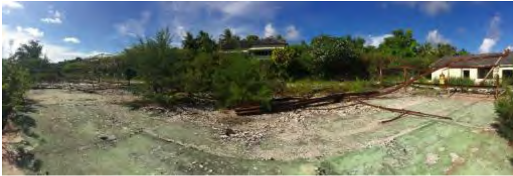
Photo 9: Warehouse 4; fire damaged structure previously containing PACM. Site covered in ACM fragments. Public roadway in background.
