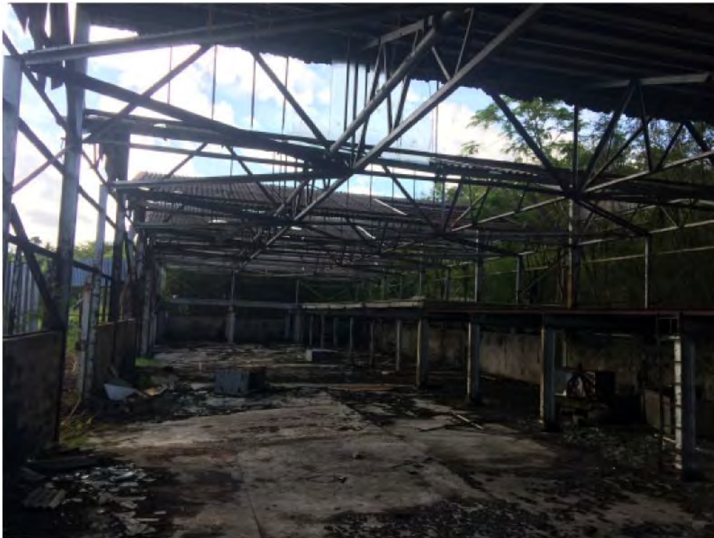
Photograph 16: Warehouse 3 – badly damaged pacm roof and walls.
