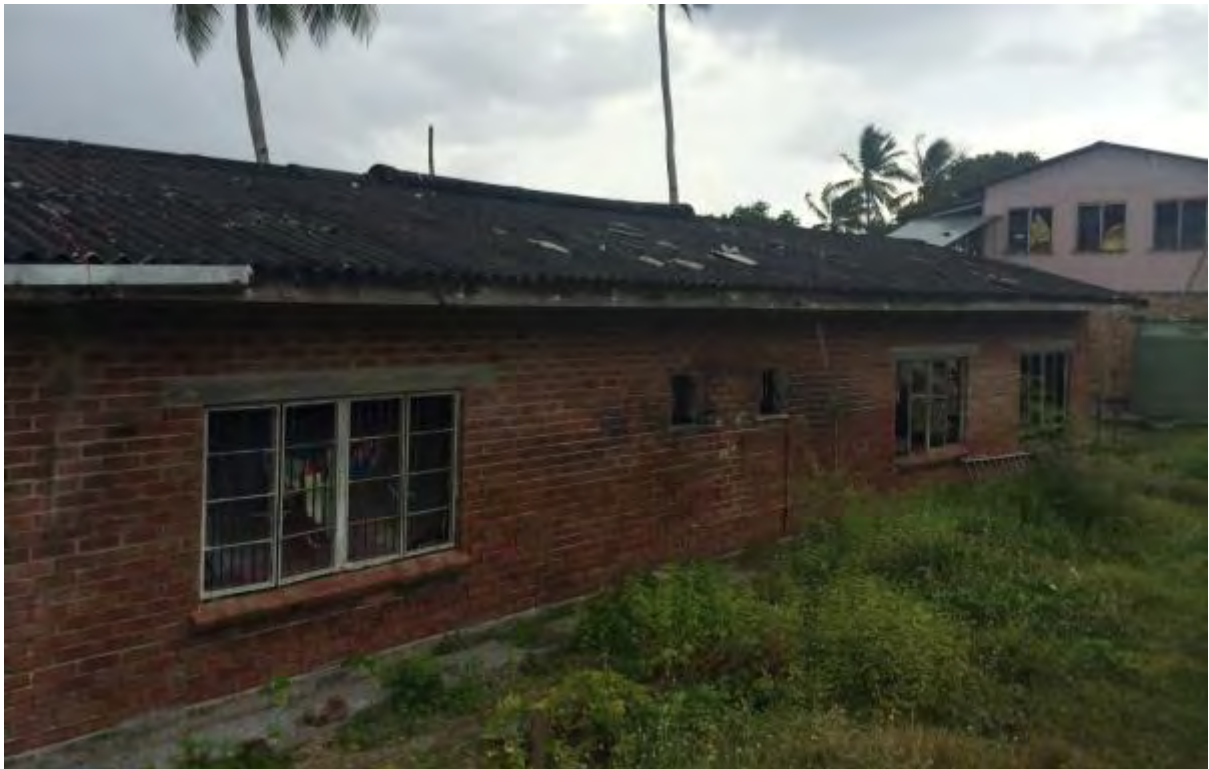
Photo 14: Banaba school, ACM roof and cladding on brick building.
