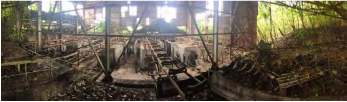
Photo 15: Former phosphate processing plant. In disrepair with significant ACM scattered across entire site.
