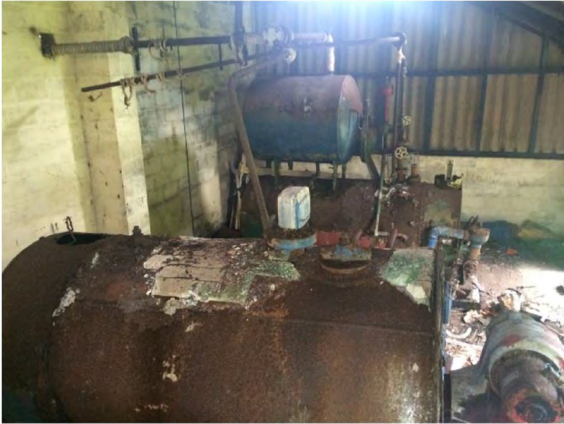
Photograph 7: Residential property 18, boilers with pacm lagging.
