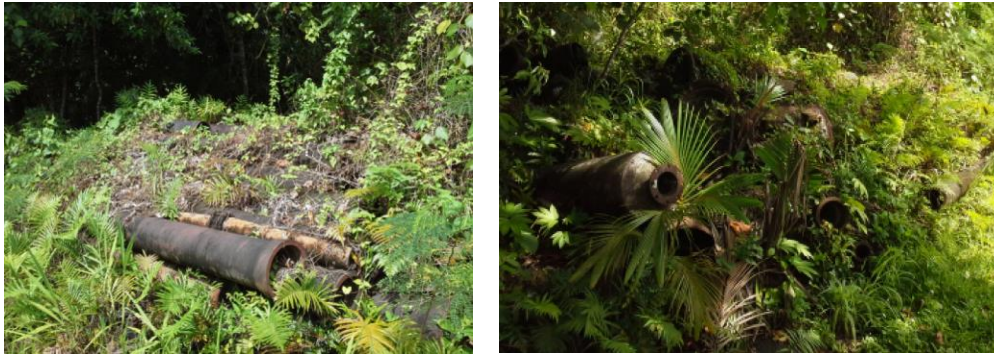
Photos 2 and 3 – Old Asbestos Pipes at Palau Water Treatment Plant
