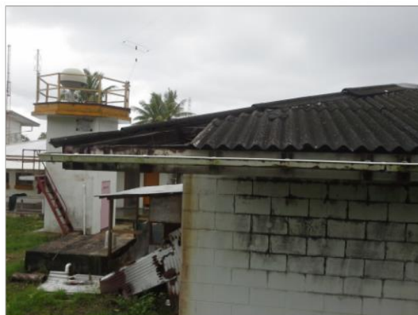
Photo 4: Asbestos roof at the meteorological centre
