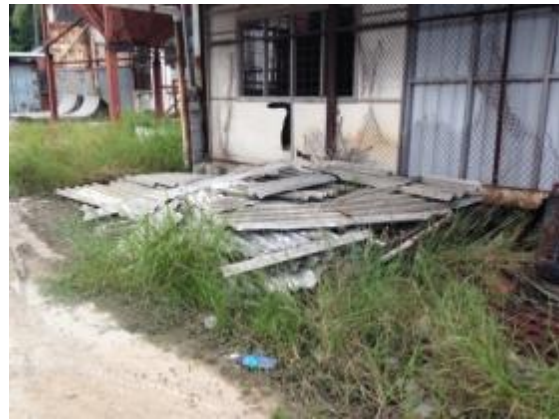
Photo 50 - Broken Asbestos Sheets
