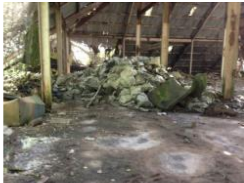
Photo 57- Abandoned Insulating Material
