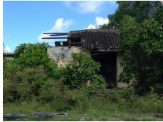
Photo 69 - Derelict Building Aiwo
