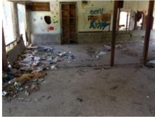
Photo 12 – Asbestos Debris in Old House
