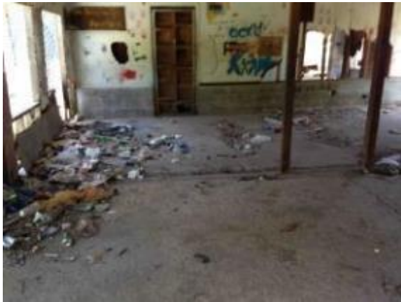
Photo 5 – Old House with Broken Asbestos
