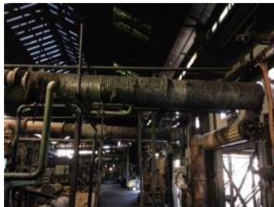
Photo 81 – Fibreglass Rope Lagging
