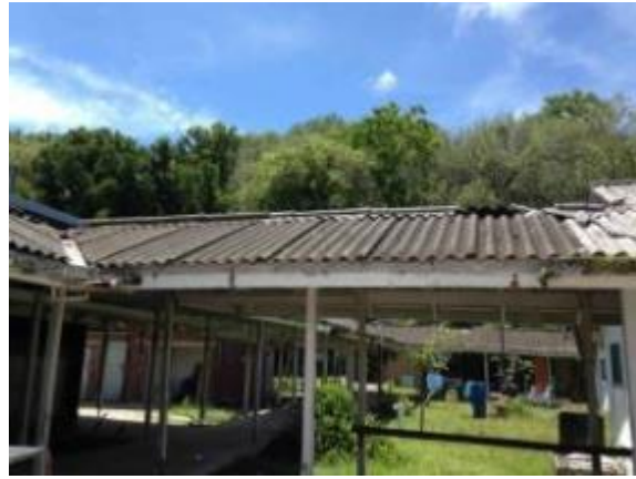
Photo 9 – Asbestos on Hospital Roofs
