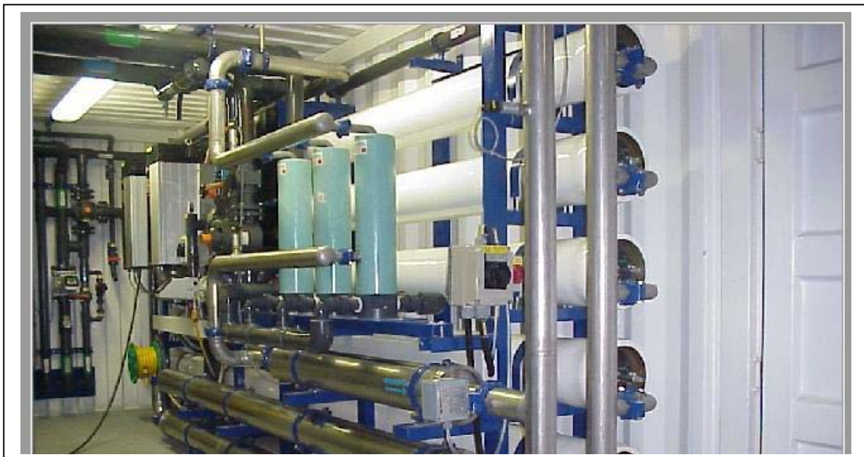
Figure 2: Typical Containerized SWRO Unit 3
