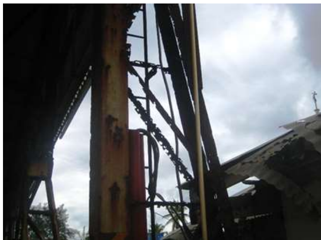
Figure 3-4: Badly corroded structural members in the Barge Shed
