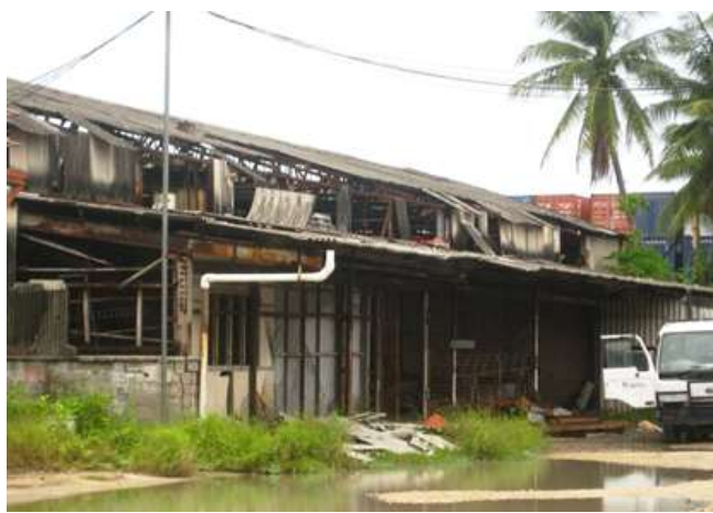
Figure 3-5: Dilapidated condition of Hardware & Bulkstore shed
