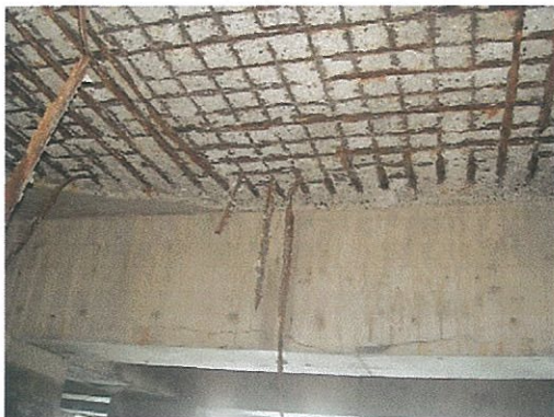
Photo-1 : Under Deck Slab Condition Almost similar situations of collapsed slab concrete. Covered concrete was peeled off and re-bar was exposed and corroded. Very danger conditions.
