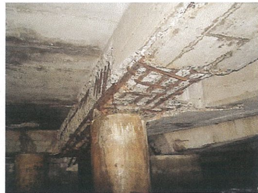
Photo-2 : Beam and Pile Head Almost all pile heads are relatively good but some part of beams are damaged and danger situations.
