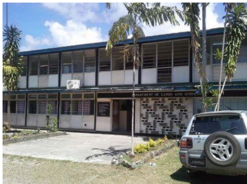
Lands & Survey Building – AC Panels
