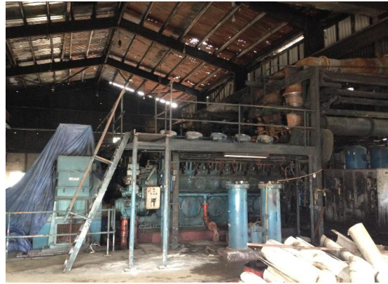
Ameliik Old Burnt-out Power Plant
