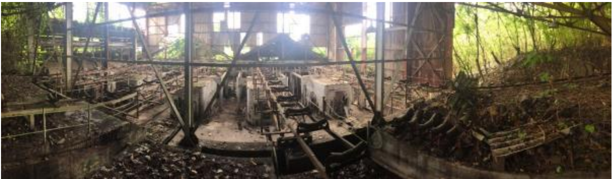
Banaba former phosphate processing plant. In disrepair with significant ACM scattered across entire site.
