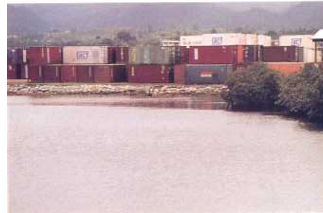
Plate 35. A seawall built to protect this reclamation close to the Port of Suva, Fiji, has failed after a short time. The mangroves that were cleared from the site would have provided better protection.
