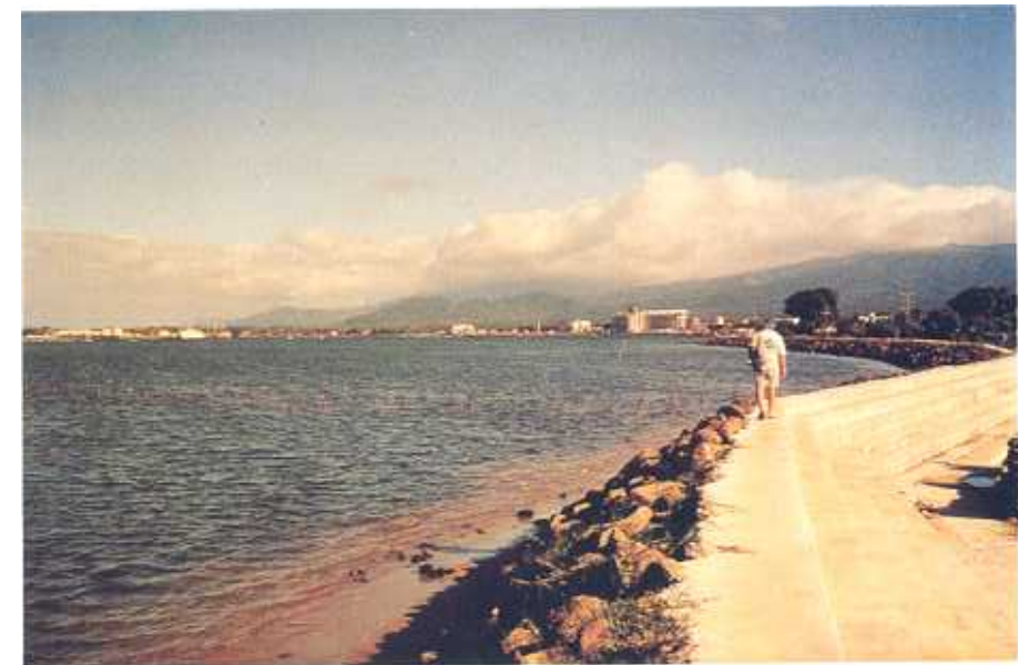
Plate 28. Designed seawall protection completed in 1994 of large boulders of volcanic rock with concrete top and walkway area behind. This structure extends from the foreground, around the two high-rise buildings on reclaimed land to the port in the distance, Apia, Western Samoa.
