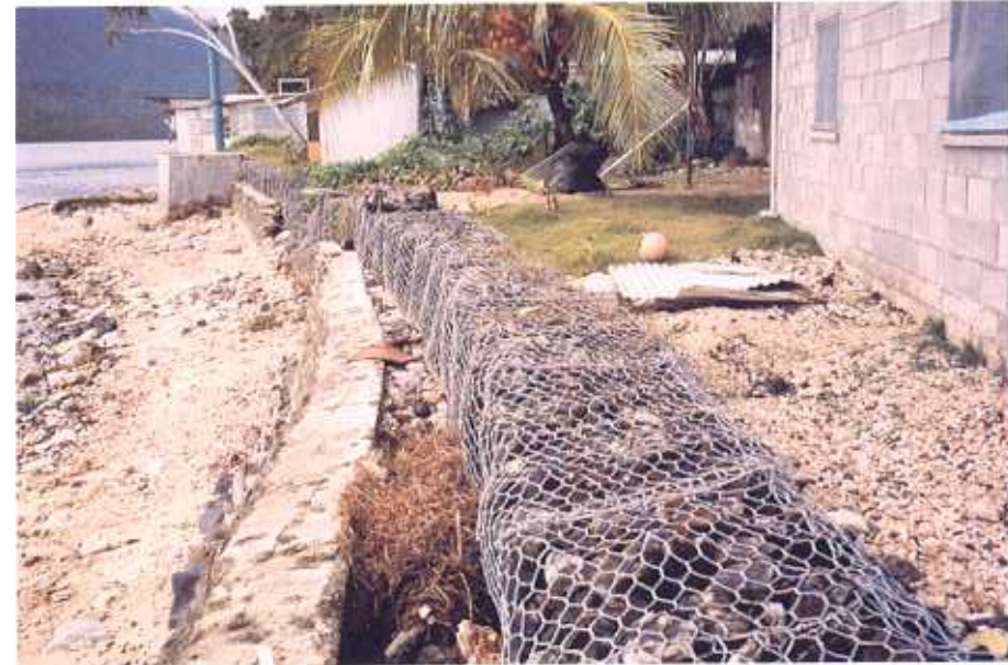
Plate 27. A repaired gabion basket seawall protecting buildings on Lelu Island, Kosrae, Federated States of Micronesia.
