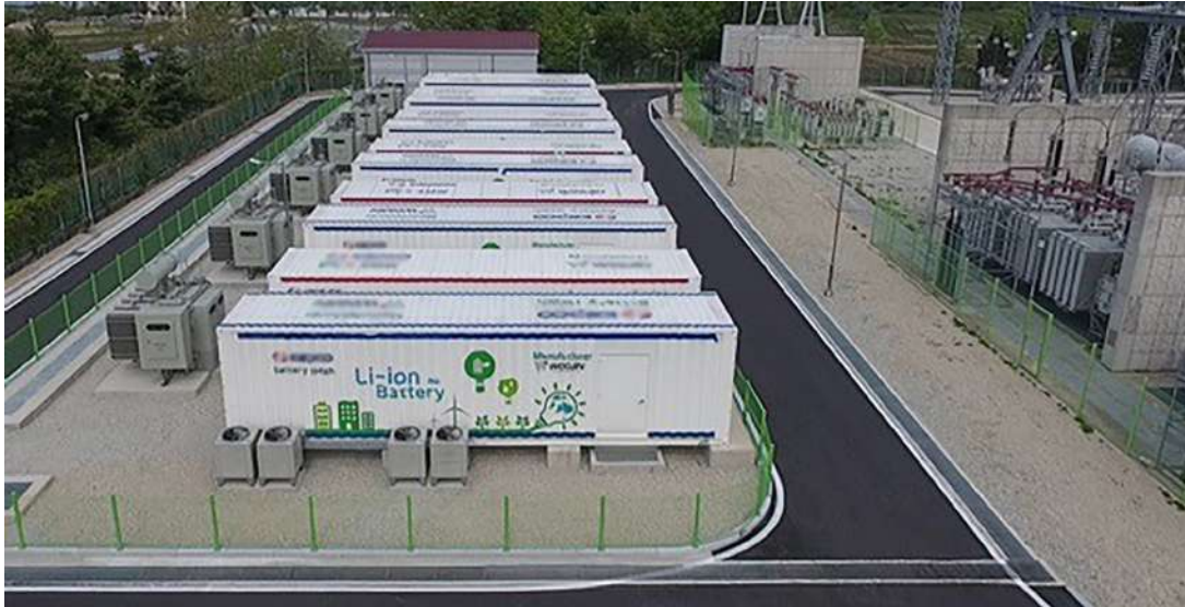
Figure D.4: Sokcho Battery Energy Storage System
