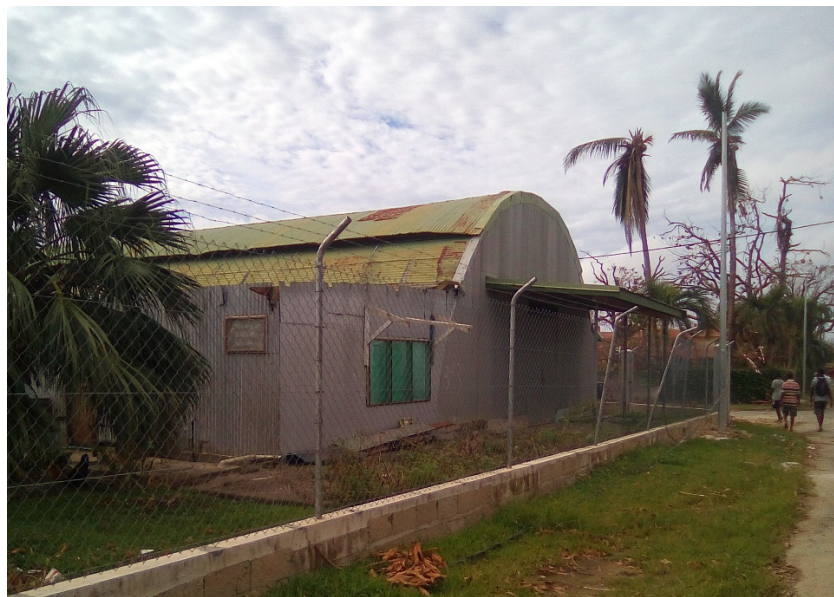
Figure 3: This building on Santo island with a curved CI sheet roof survived the cyclone (source: Renata Netaf).
