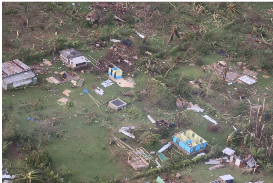
Figure 1: This aerial photo shows houses that lost their CI sheet roof in the cyclone; the house in the top left with a RC roof survived (source: Tony Deamer).
