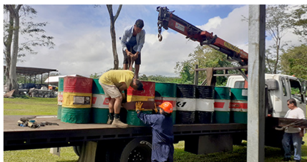
Wrap the belt around the crane and wrap it around the waste oil drum to secure it.
