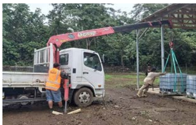
First unload of waste oil to SWOMP facility, February 2021
