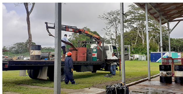
Lift up the waste oil drum secured by belt.
