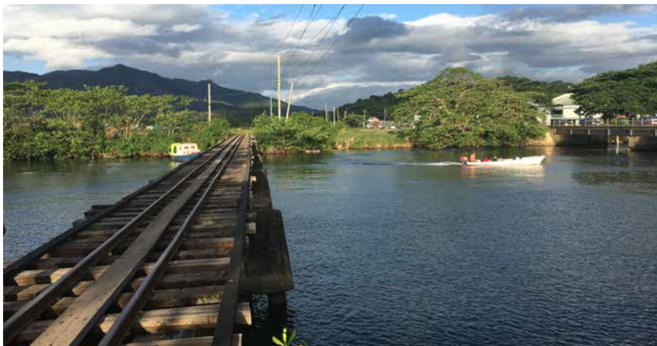
Tramline across Labasa river, Macuata Province. Transportation and energy infrastructure are particularly vulnerable to storm, flood and erosion events. Photo: WPN.
