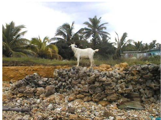
Fig. 9 Part of the degraded seawall protecting the village of Yadua—storm waves penetrate into the land behind the damaged sea wall and erode the coastal flat on which the village lies (Photo: Patrick Nunn, Fiji)
