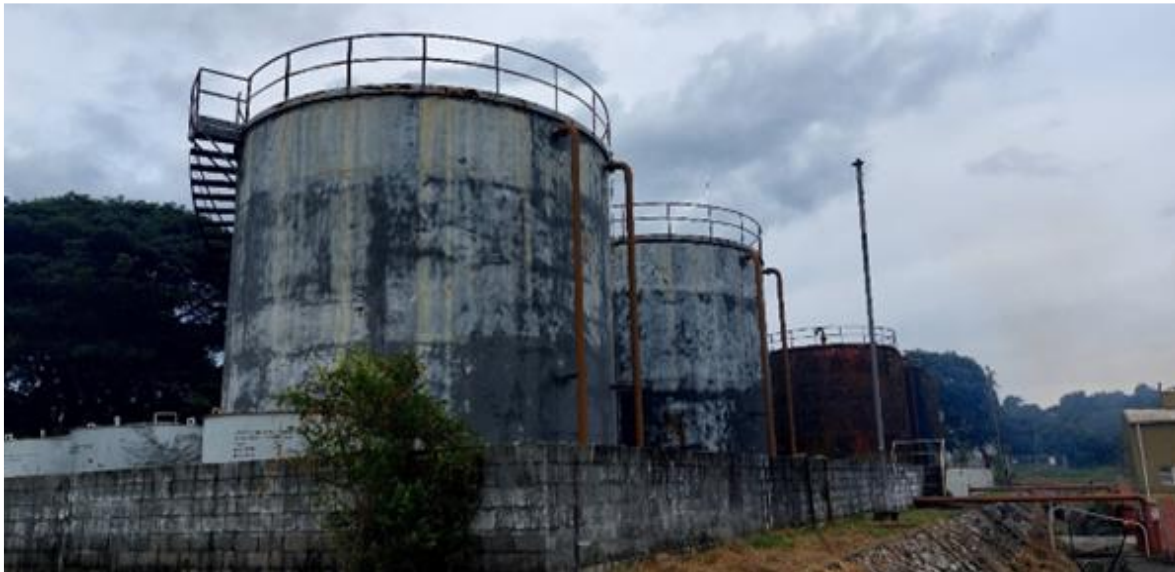
Figure 4: PCB contaminated oil is stored in Tank 1 estimated at 400 000L. The tanks are in a bunded area.
