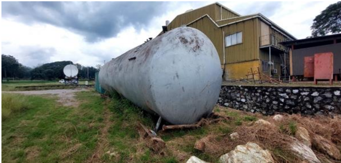
Figure 5: The remaining 20,000L of PCB contaminated oils are stored in this tank that is outside in the yard.
